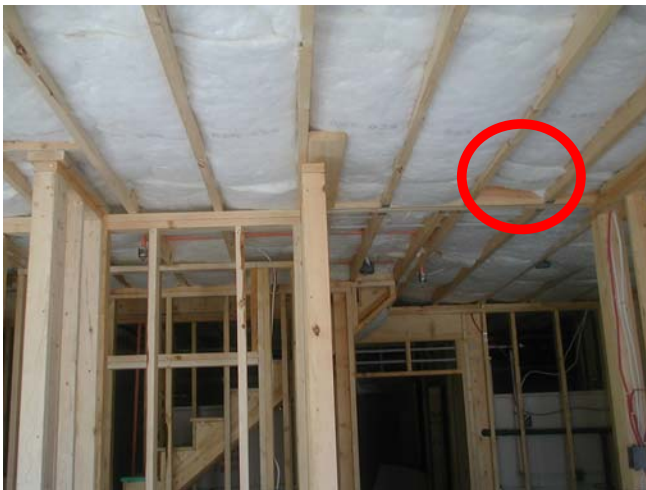
Figure 1.6 - Insulation installed with gaps and voids
