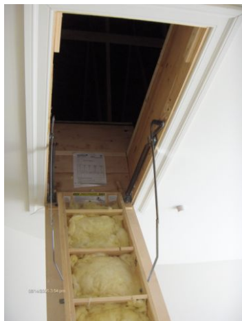
Figure 5.2 - Improperly installed insulation impedes use of drop-down attic access stair
