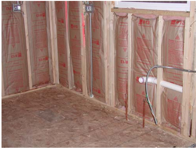
Figure 1.5 - Insulation installed with voids and compressions
