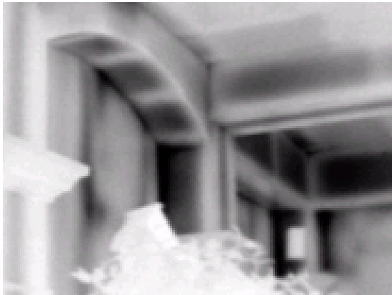
Figure 10.2 – Infrared image of poorly insulated dropped ceiling
